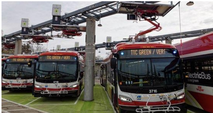
Figure 3: Electric Buses at a Toronto Transit Commission (TTC) Charging Station
